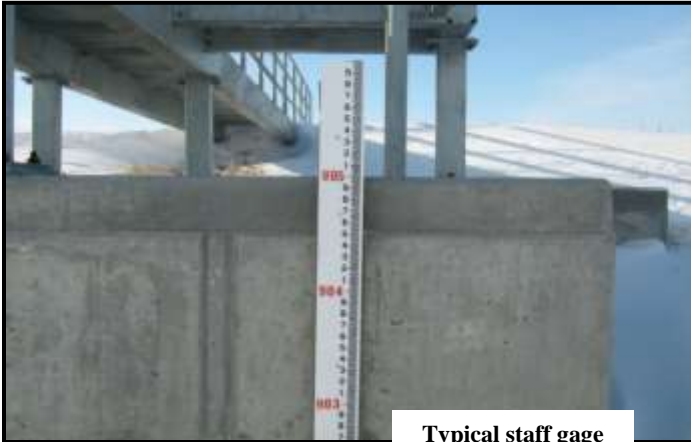
Typical staff gage at structure
